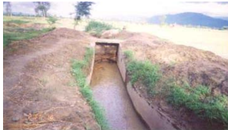
Figure 2: Intake Structure of Baireni Canal Constructed by Using Stone filled Gabbion Boxes
