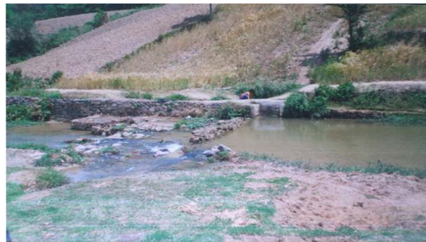
Figure 5: Intake with Combination of Gabion and Core Wall Diversion of Harishidi Irrigation System, Lalitpur District
