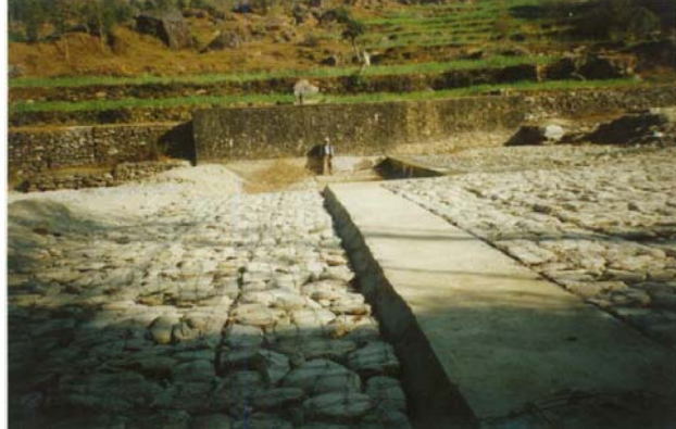
Figure 6: Bottom Rack (Tyrolean) Intake, Myagdi District
